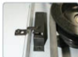
Micro-Switch on Pulley Guard
